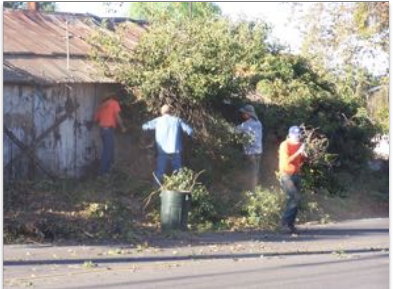
Work party clearing brush from the building in South Ontario in preparation for the removal of the 160HP Western engine.
